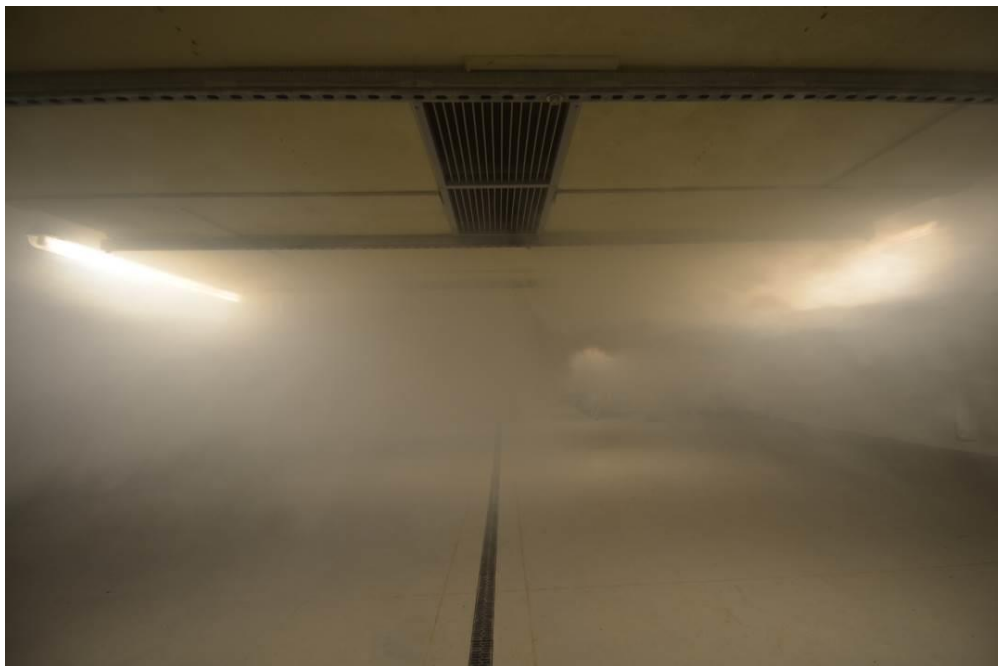
Fig. 7 Inefficient operation of a mechanical smoke extract system in a car park due to positioning of the extract grille at the bottom of the smoke duct
